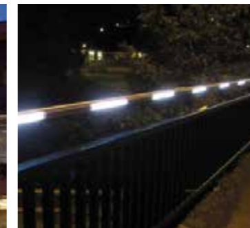
Solar handrail lighting
